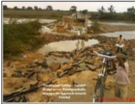
Bridge damage Dharwad district – 5 th October 2009
